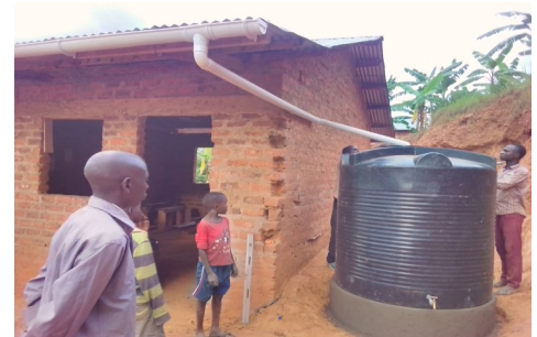
Rain water harvesting system and water tank
